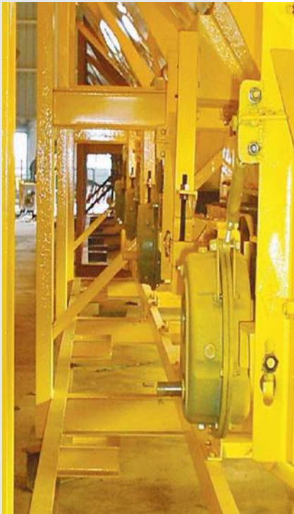
Shaft mounted drive in Conveyors
