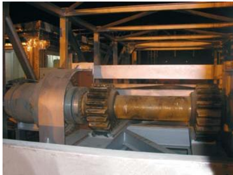
Coke pusher drive
